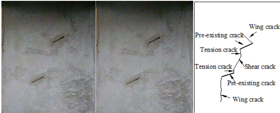
Fig. 10. The transfixion pattern of wing cracks under the tension-shear combined failure mode.
